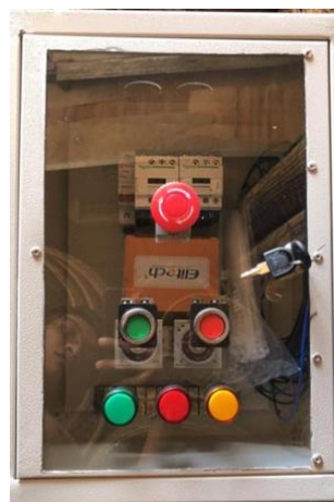
Gambar 5. Panel kontrol sistem automatically cooling and defrost system
